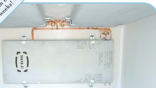
COLD PLATE REFRIGERATION SYSTEM
